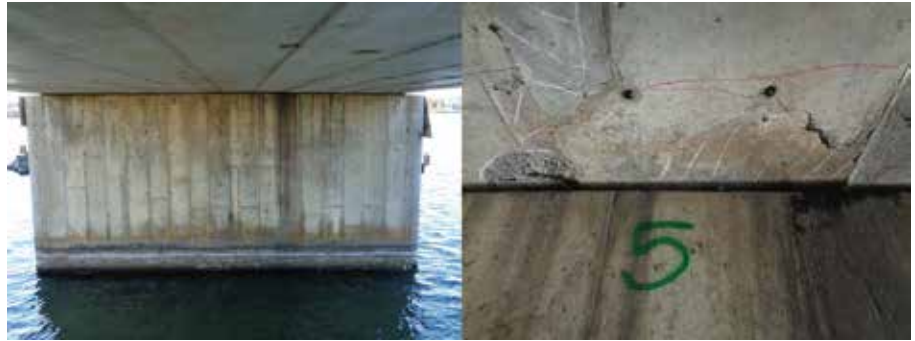
Fig. 6: The underside of the LaSalle Causeway bridge deck exhibited visible damage only near the central pier
