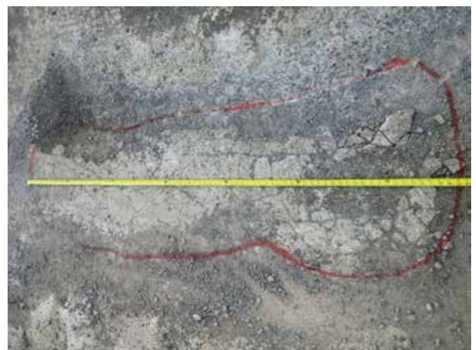
Fig. 3: An example of a damaged area on the Three Nations Bridge
