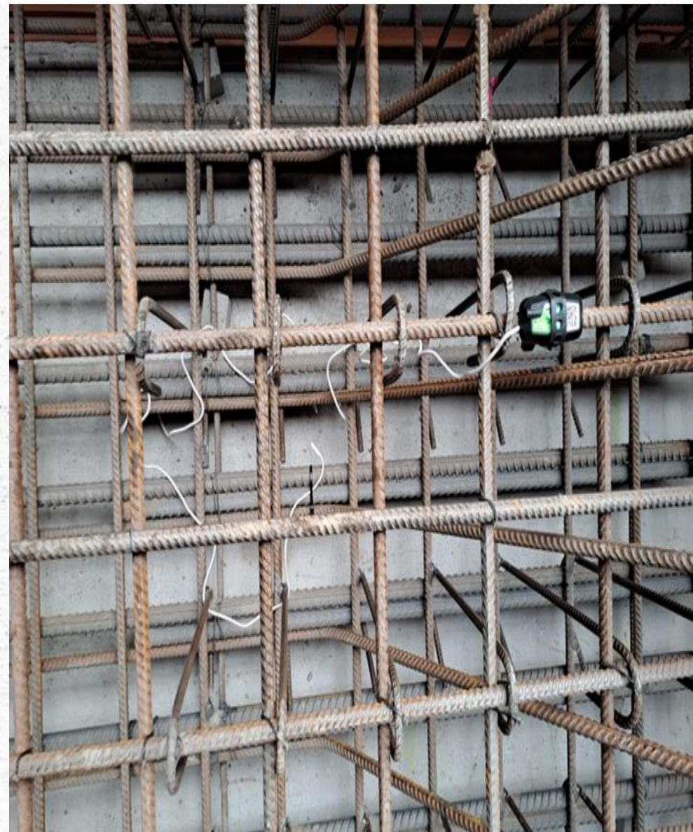
Bad Installation – Cable not securely attached to the rebar
