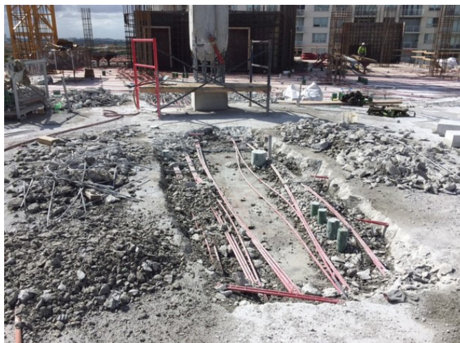
Figure 6-4: Example of damages due to early post tensioning
